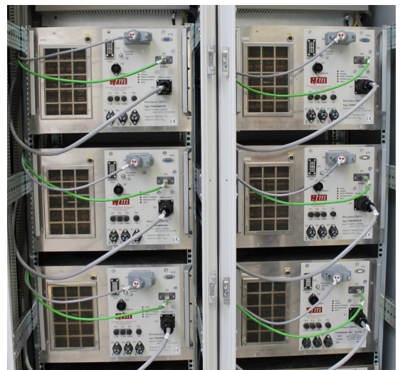
Cabinet with Switch Mode Power Supplies
